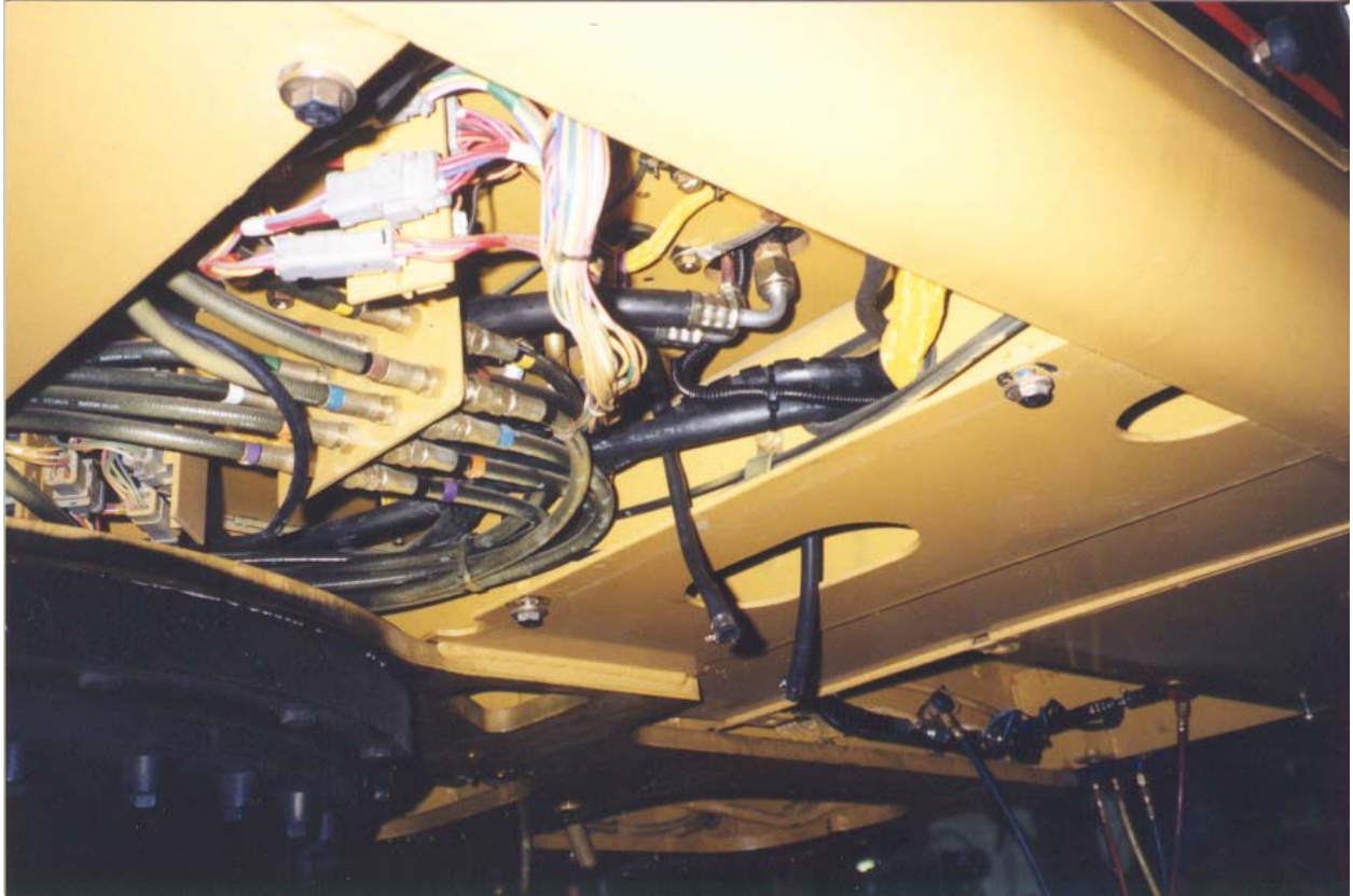
View showing underside of evaporator area with hose assemblies.
